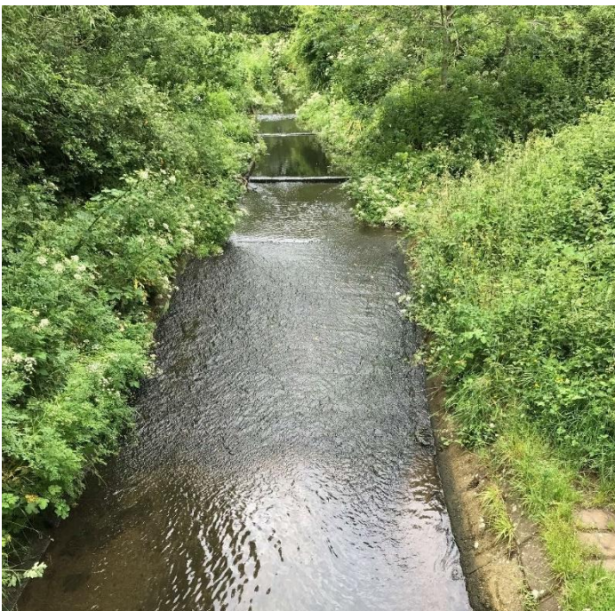
Graphic 3-2 An upstream view of the sloping weir with masonry face followed by a vertical weir with smooth concrete crest within Hermitage Stream
