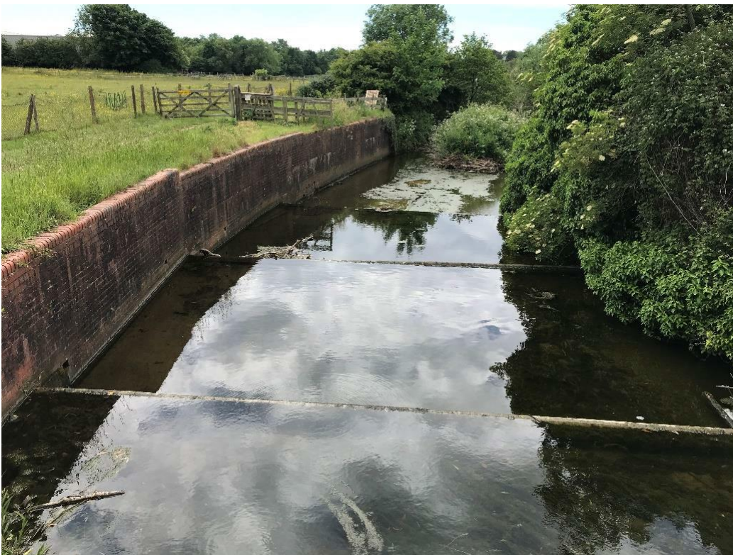
Graphic 3-4 Sequence of three step weirs within Hermitage Stream (photo taken looking downstream)
